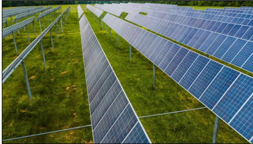
Figure 15: A Typical Operational Solar Farm (Credit: Energy Guide UK 34 )
